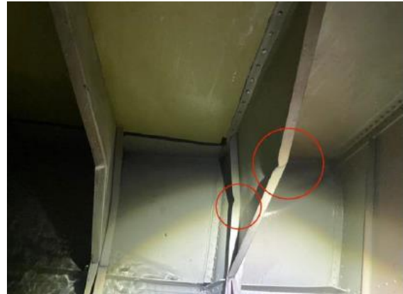
Figure 8: Right hand side panel (PN: 1011235) of number 8 bulkhead torn
