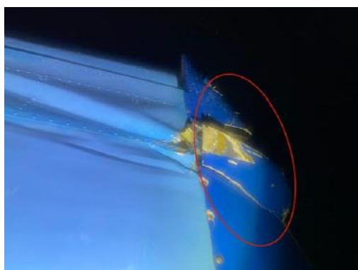
Figure 5: Left wing tip fairing (PN: C6W1004-1) damaged
