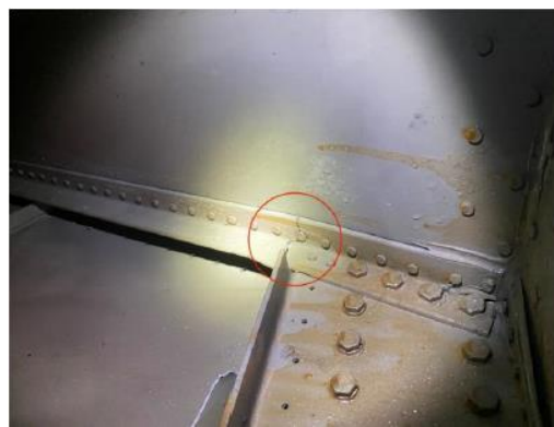
Figure 2: The left hand inboard AFT stiffener (ARM, PANEL, RH, #6 BULKHEAD, PN: 13A01427-010) of the number 6 bulkhead has been cracked
